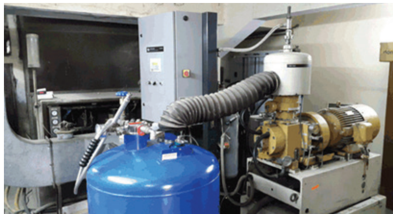
Figure 2 : Liquid Nitrogen Facility
